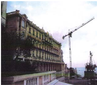
Sight of the Hotel Hermitage. 16 triaxiaux sensors were installed on the architectonic structures of the building
